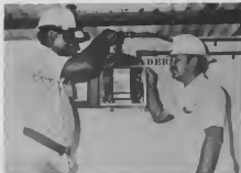
Project Leader Pat Kock observes how Ernie Williams calibrates Flow Meter Amplifier which powers the flare probe at the stack.
